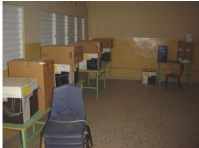
Some labs remain in boxes after four years due to a lack of connection to the electricity grid.
